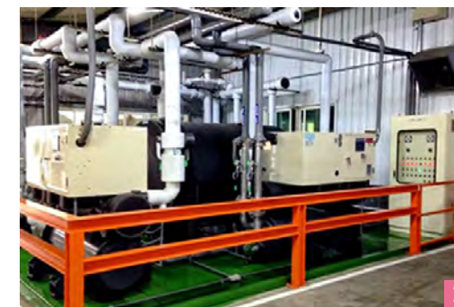
1 製程水回收設備 Process Water Recycled Equipment
