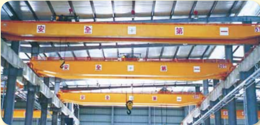
一般廠房（鋼鐵廠）使用 Hoist in Steel Mill Application ( 20 ton Wire Rope Hoists for high frequency lifting )
