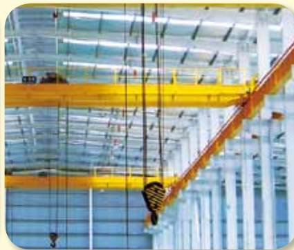
一般廠房（鋼鐵廠）使用 Hoist in Steel Mill Application ( 20 ton Wire Rope Hoists for high frequency lifting )
