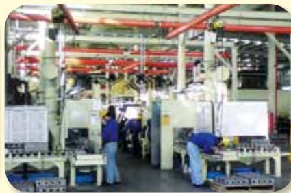
一般廠房（鋼鐵廠）使用 Hoist in Steel Mill Application ( 20 ton Wire Rope Hoists for high frequency lifting )
