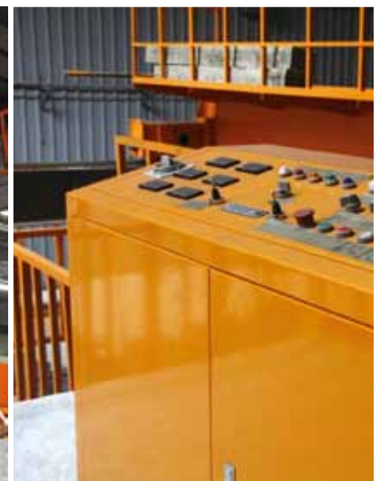
Hoist Electric Testing ( 電路測試 )
