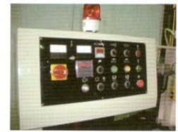
電控系統 Electric control system
